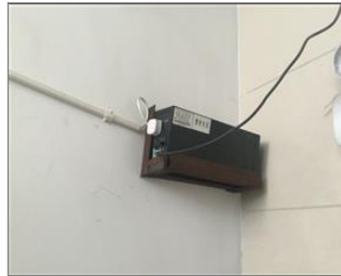
Photo of fire safety equipment backup power.JPG
